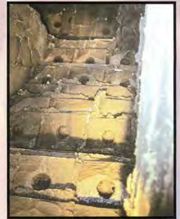
Jagged Corbelling and Exposed Brick Cores (Holes) in a Smoke Chamber
