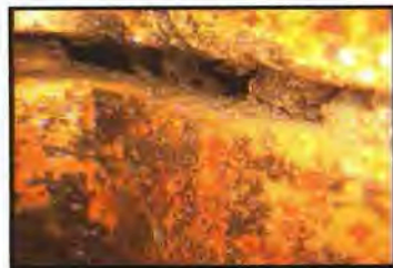
Actual photo of deteriorated mortar joint between flue tiles
